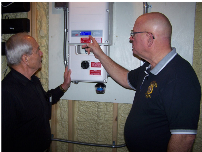
Bill Decker and Bob Schmitt check out the solar inverter in the basement of the Schmitt home that indicates how much energy the solar panels are generating. Toledo Free Press photo by Duane Ramsey
